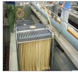
MBR in Qishuyan WWTP
